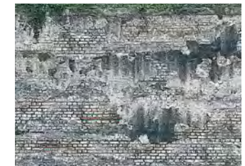
H0 TT 7415 Verwitterte Industriesteinmauer Weathered industrial wall. Mur industrielle.
